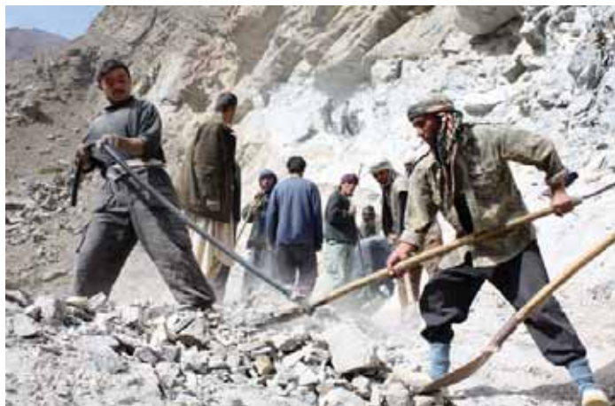
New roads facilitate trade and transportation and the road construction employs many people. Photo: UNAMA
